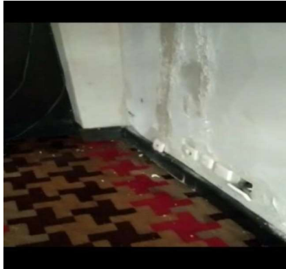
Gambar 4 Dinding Meeting Room Rusak
