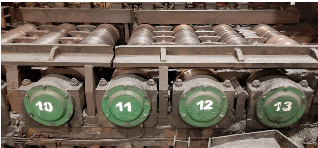
Lampiran 6. Gambar Working Roller Table di PT. Krakatau Steel Divisi Hot Strip Mill (HSM)
