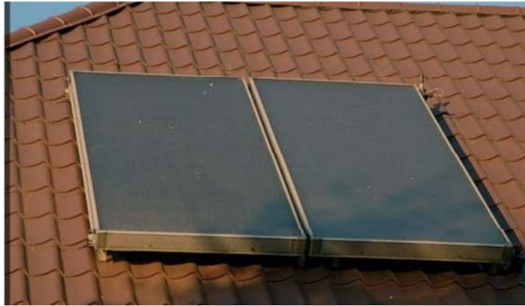
Gambar 1. Solar water heater
