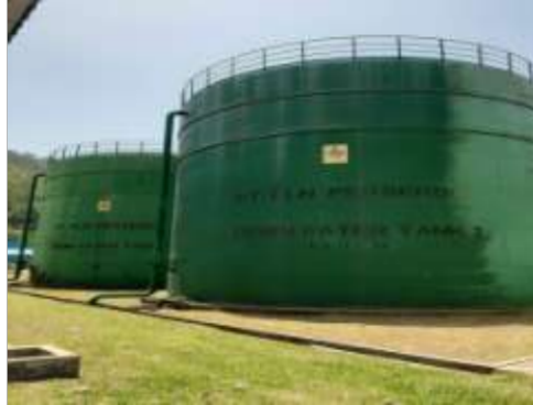
Gambar 32. Demin Water Tank.
