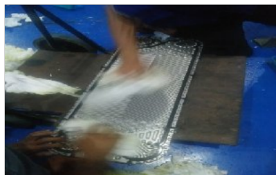
Gambar 4.2.7 pengeringan Plate Heat Exchanger
