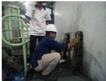
Gambar 4.2.5 pembersihan Plate Heat Exchanger
