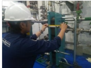
Gambar 4.2.10 pengukuran jarak Plate Heat Exchanger
