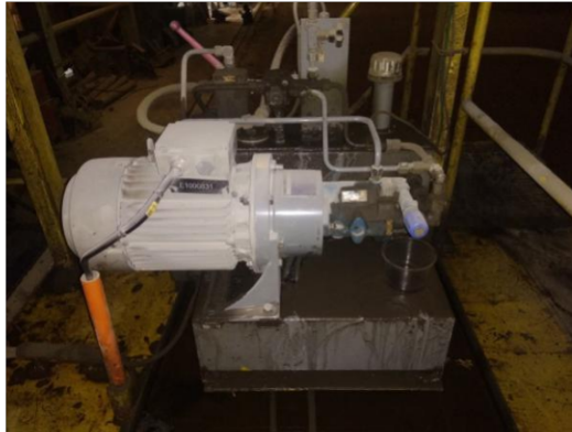
Gambar 12. Hydraulic Pump Station (Sumber : Dokumentasi Pribadi)
