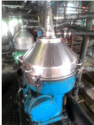
Gambar 2.11. Sludge Separator (Alfa Lafal)
