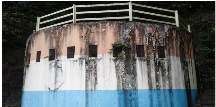
Gambar 1.6. surge tank PLTA Batang Agam
