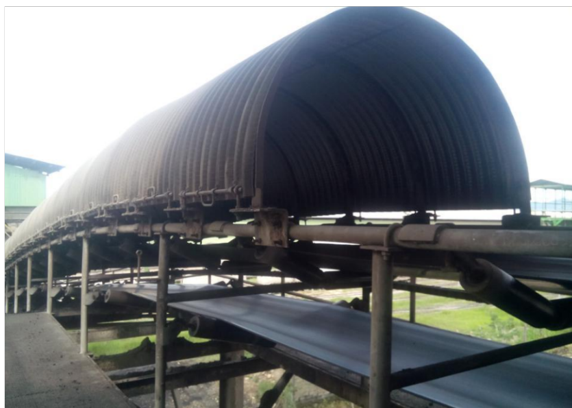
Gambar 2. 1 Belt Conveyor Batu bara
