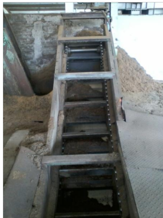
Gambar 20. Recycle Scarper Conveyor
