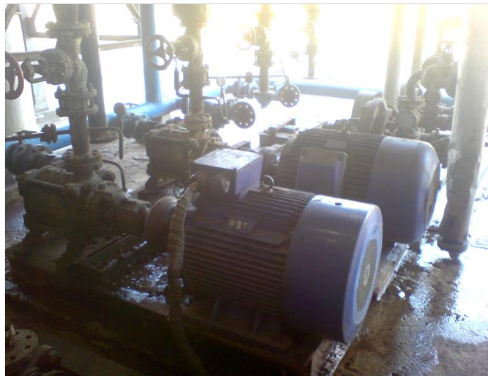
Gambar 13. Boiler Feed Pump
