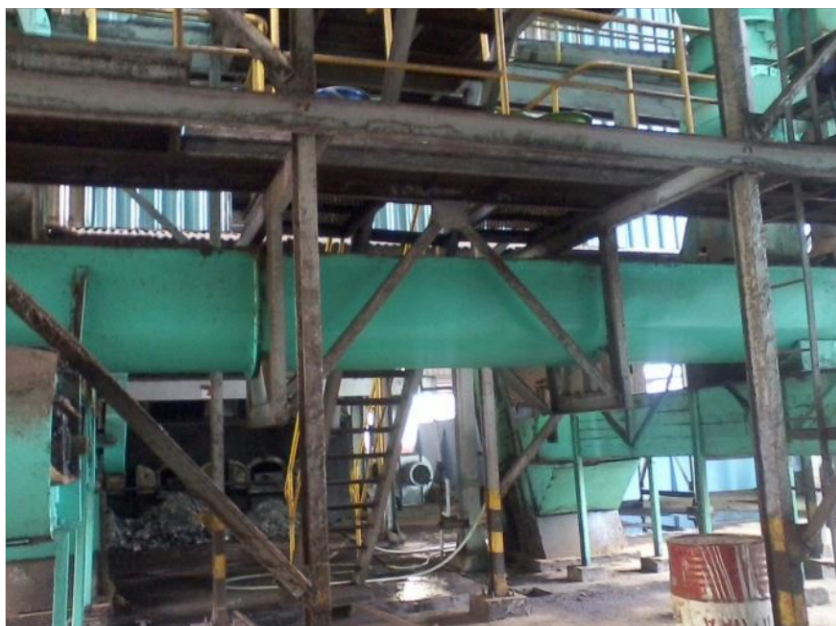
Gambar 15. Fiber and Shel Cross Conveyor
