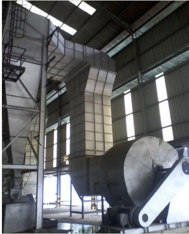
Gambar 24 . Induced Draft Fan
