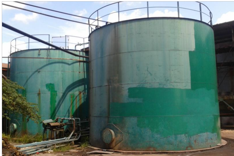
Gambar 11. Feed Water Tank
