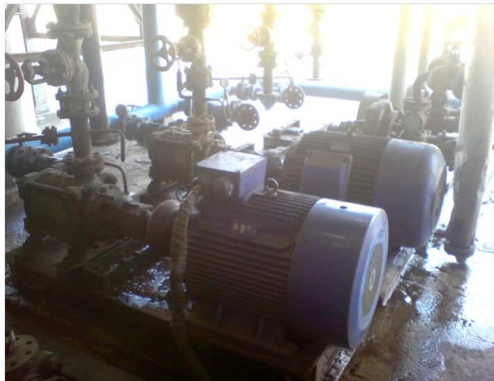
Gambar 13. Boiler Feed Pump
