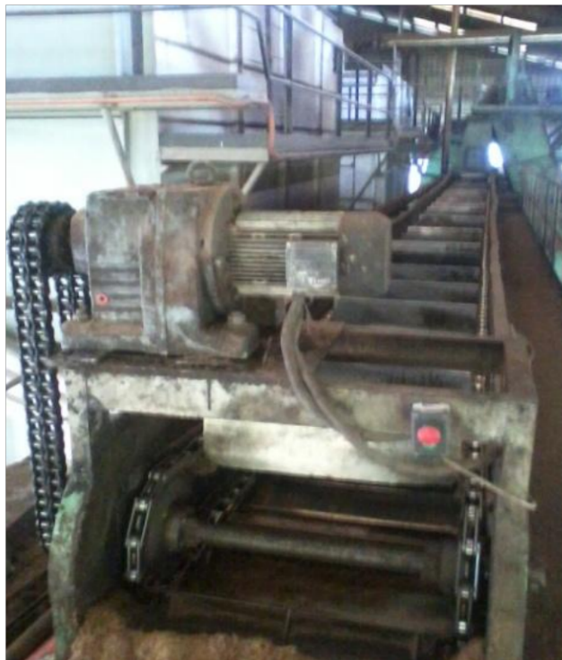
Gambar 18. Fuell Feed Scraper Conveyor
