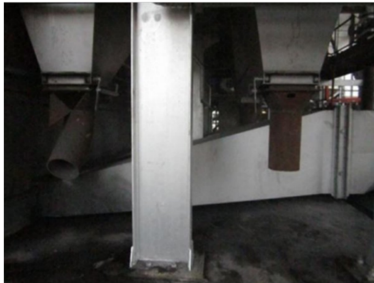
Gambar 9: Pembuangan Abu (Ash Hopper)
