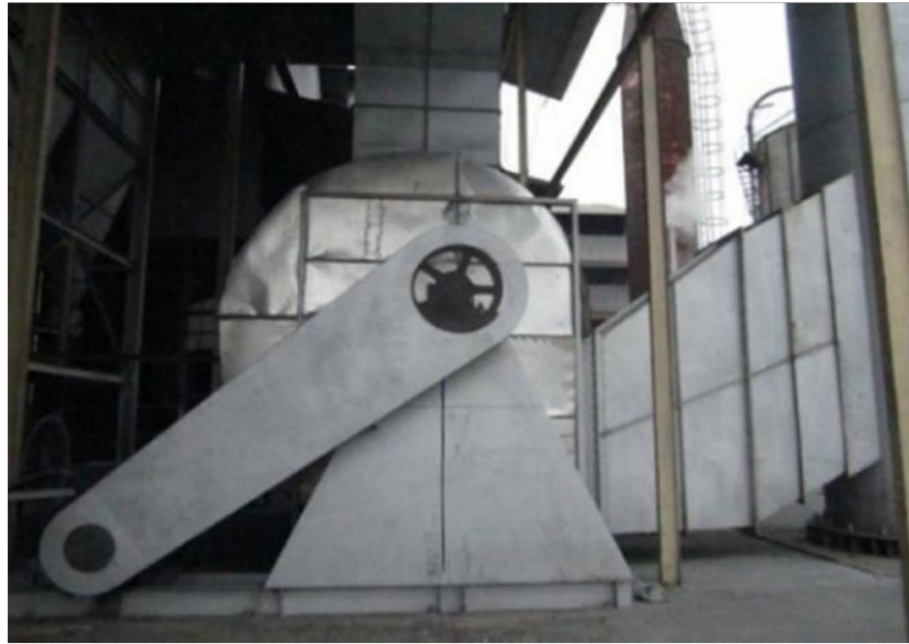
Gambar 12: Induced Draft Fan
