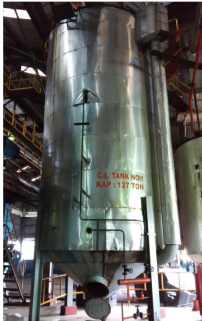
Gambar 2.13 Continous Settling Tank
