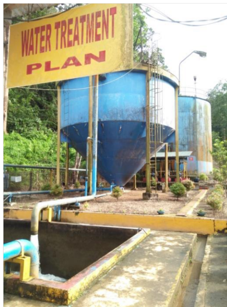
Gambar 2.29 Water Treatment Plant
