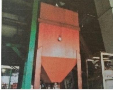
9. Sand Trap Tank
