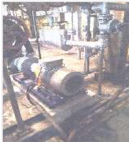
Gambar 3.13 Boiler Feed Water Pump
