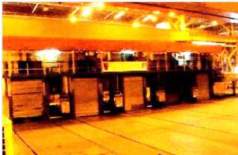
Gambar 3.6 Line Continuous Tandem Cold Mill
