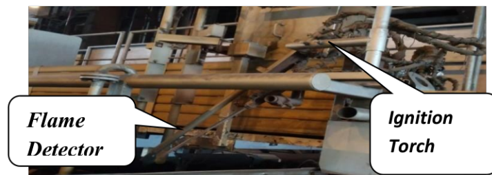
Gambar 33. Electrical Ignition torch dan Flame Detector
