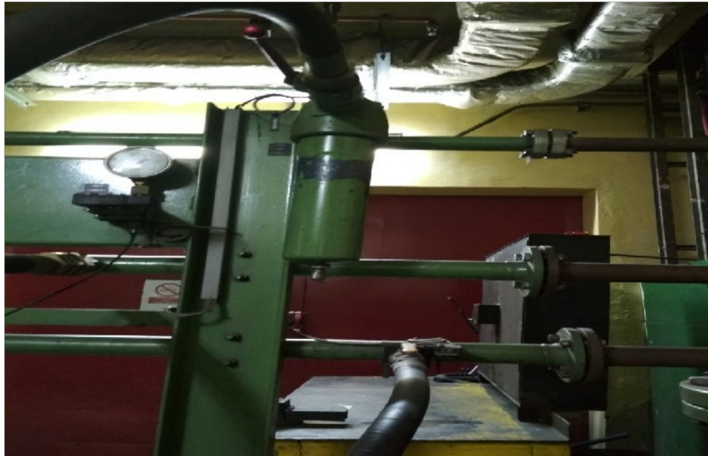
Gambar 5.7 Filter Pompa High Pressure
