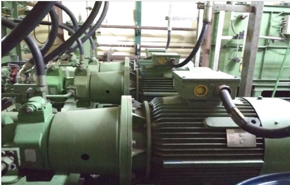
Gambar 5.3 Pompa High Pressure
