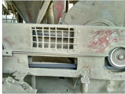
Gambar 4.3 Pulley dan V-Belt (Sumber: Bagian Area Jet Pulse filter, air sluice, apron conveyor, Indarung V PT. Semen Padang)
