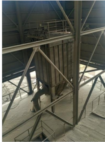
Gambar 4.1 Jet Pulse Filter (Sumber: Bagian Area Jet Pulse filter, air sluice, apron conveyor, Indarung V PT. Semen Padang)
