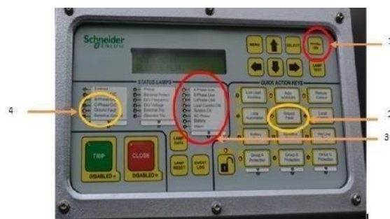
Gambar 4. Panel Kontrol Recloser
