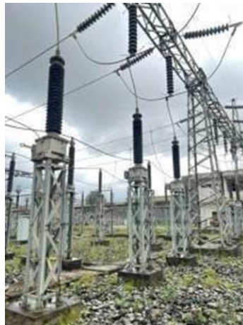
Gambar 2.3 Foto Capacitive Voltage Transformer
