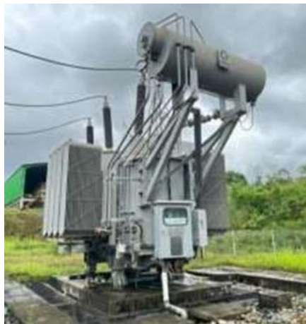
Gambar 2.1 Foto Trafo Daya 30MVA,150kV/6,3kV
