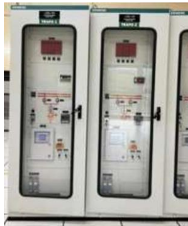
Gambar 2.6 Foto Control Panel
