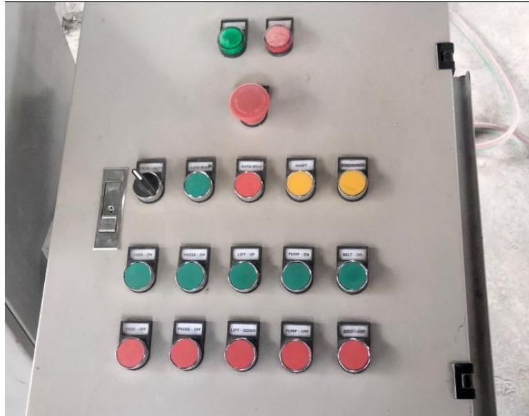
Gambar 4.20 Panel Control Desk Mesin Interlock brick
