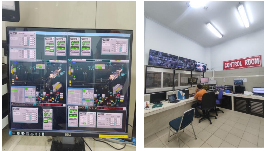
Gambar 3.12 Monitoring dan Control Room
