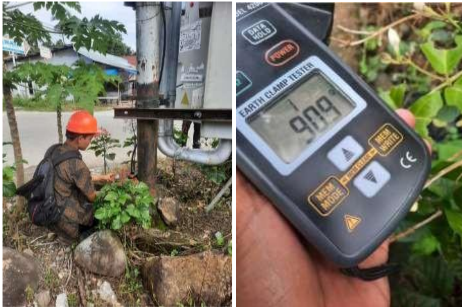
Lampiran 3 Pengecekan Pentanahan Arrester
