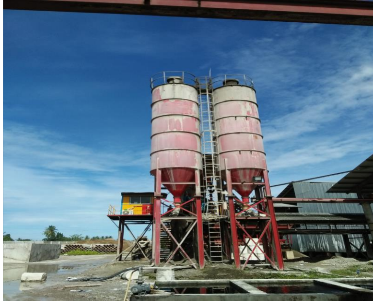
Gambar 11. Batching Plant Sumber . PT Jaya Sentrikon Indonesia
