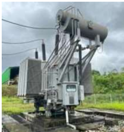
Gambar 2.1 Trafo Daya 30MVA,150kV/6,3kV
