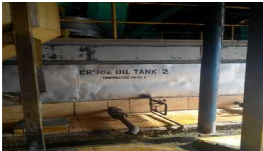
Gambar 11. Crude Oil Tank
