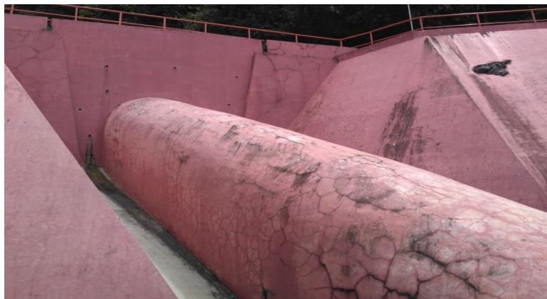
Gambar 2.5 Penstock PLTA Batang Agam
