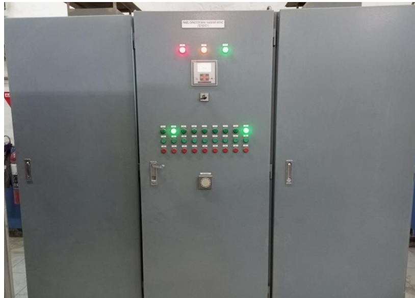
Gambar 15. Panel Kapasitor Bank Low Voltage
