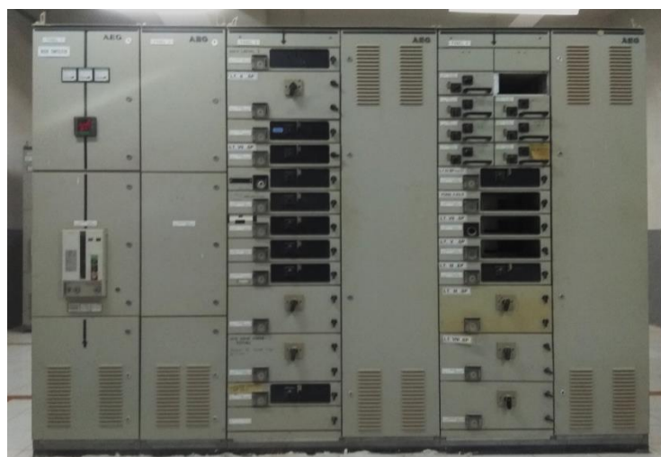
Gambar 14. Non Process Distribution Board (NDB)
