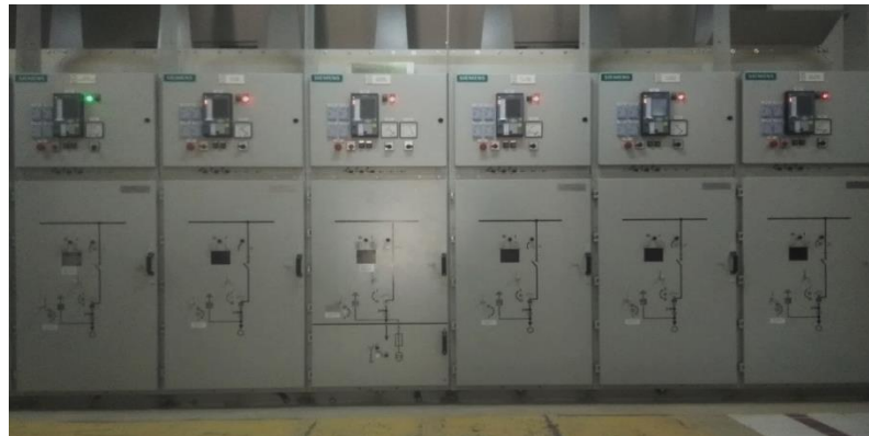
Gambar 8. High tension distribution board (HTDB)
