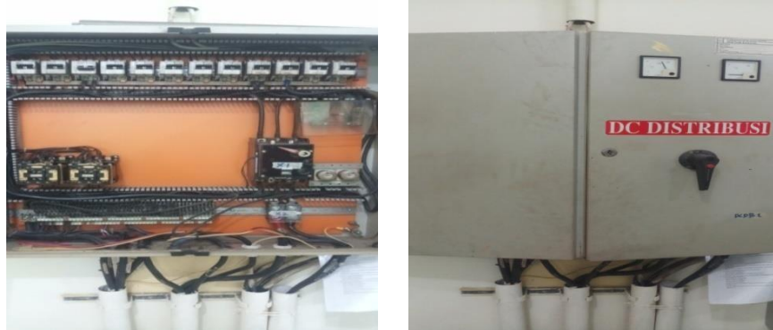
Gambar 4.9 Panel Distribusi DC (Sumber :Gardu Induk Solok)
