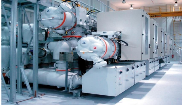
Gambar 3.2 Gas Insulated Switchgear
