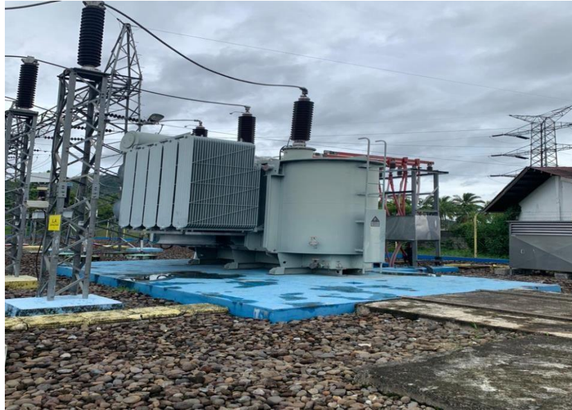
Gambar 3.9 Transformator Daya 2 60 MVA
