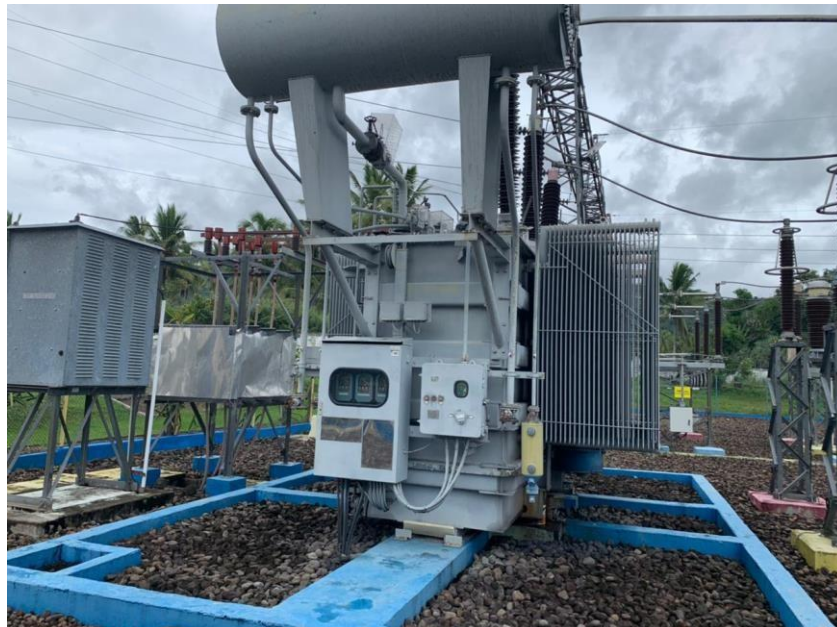
Gambar 3.8 Transformator Daya 1 20 MVA
