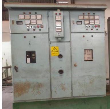
Gambar 2. 5 Panel sub distribusi
