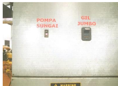
Gambar 2. 7 Panel kontrol motor
