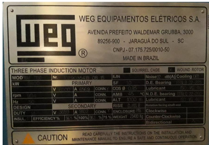
Gambar 9 Nameplate Motor Mill 6Z1M03
