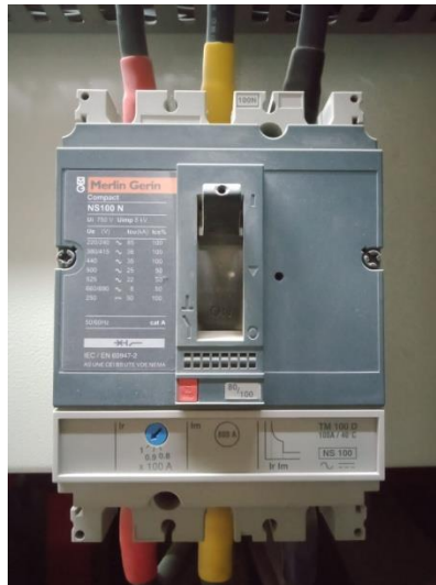
Gambar 38. Main Circuit Breaker
