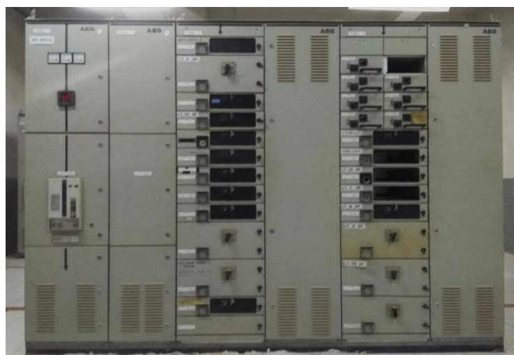
Gambar 14. Non Process Distribution Board (NDB)
