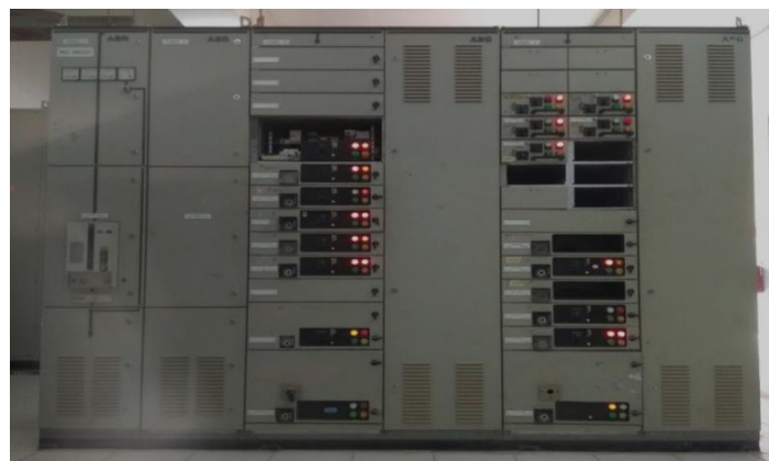
Gambar 12. Motor Control Central(MCC)
