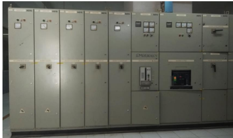
Gambar 10. Main Distribution Board (MDB)
