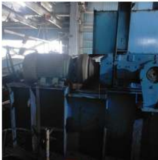
Gambar 8: Motor Belt Conveyor di PT PLN INDONESIA POWER UPK Teluk Sirih
