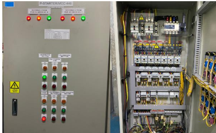
Gambar 2. 6 Panel DOL Starter MCC 446 Utility
