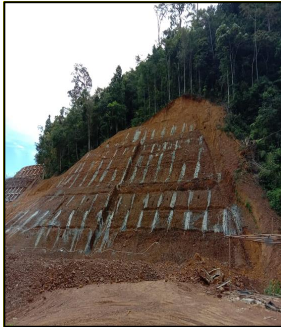
Gambar 2. Kondisi Lereng Area 8 PT. Dairi Prima Mineral
