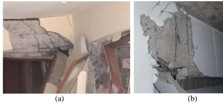
Figure 1. Typical shear failure on beam due to seismic loading : (a) in Turkey, 2003; (b) at The Grand Chancellor Tower in South Island, NZ, 2011 http://www.koeri.boun.edu.tr ; http://db.concretecoalition.org
